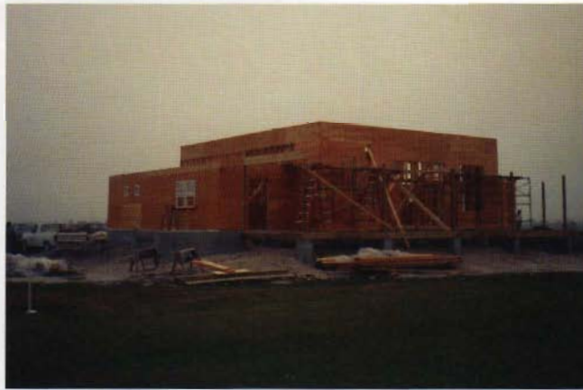
^ The Sarasota Polo Clubhouse under construction in November, 1992 The Pavilion would start the following year, September 1993
